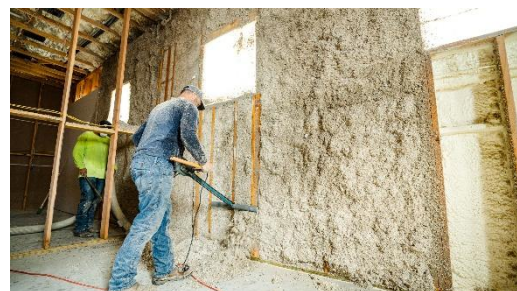
Figure (2-8) Cellulose Insulation
