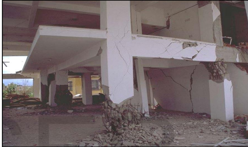
Fig. 1.3 Short columns failed (Games and Musa, 2016).
