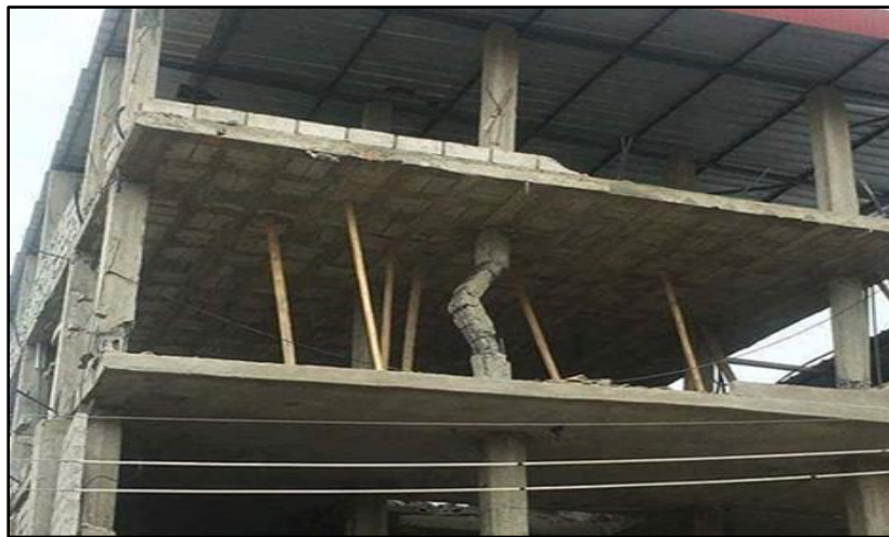
Fig. 1.4 Buckling failure (Module, 2017).
