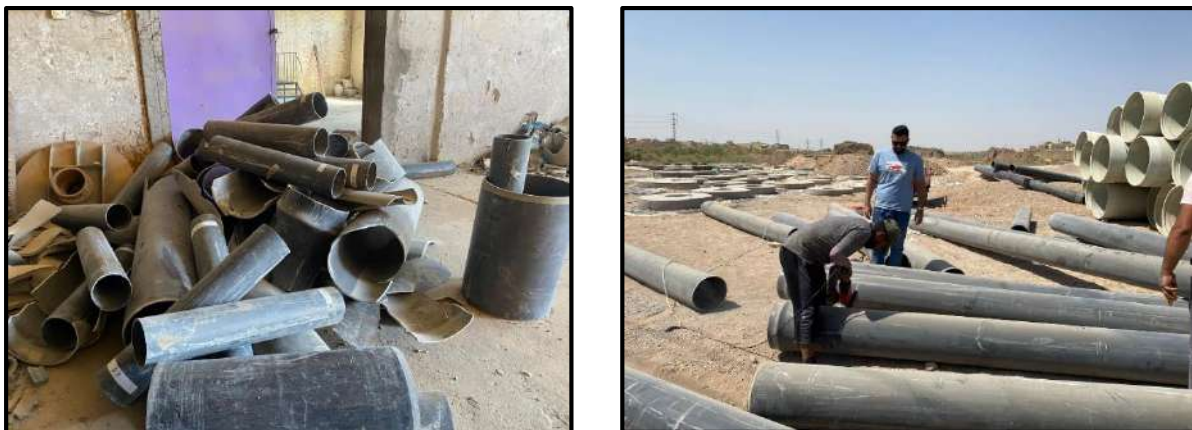
Figure 3.4 Unwanted PVC Pipes
