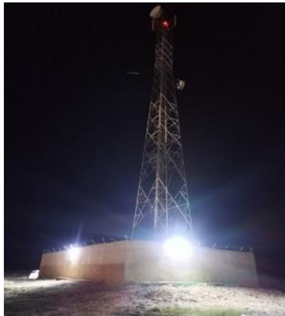
Figure 3-12. UMTS for Site 3 .
