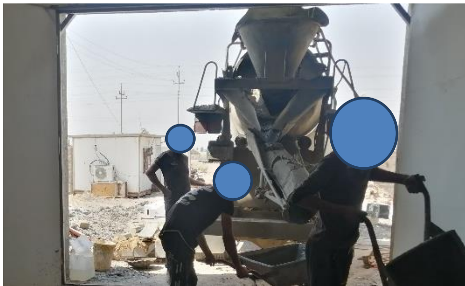
Figure 3.17 Mixer of concrete
