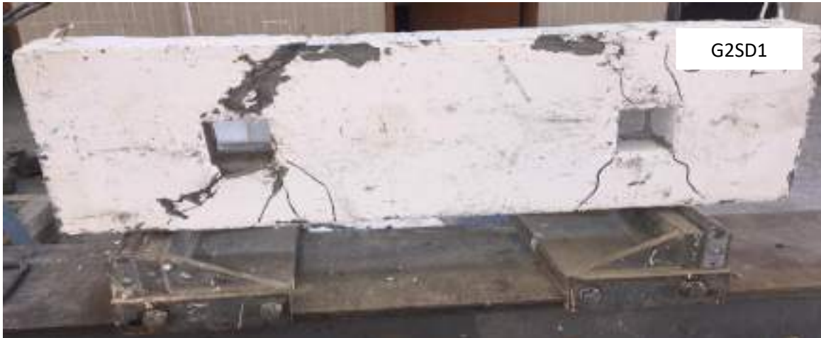
Plate (4.33b) Experimental Deep beam (rear view) G2SD1 (9%SF) after failure.
