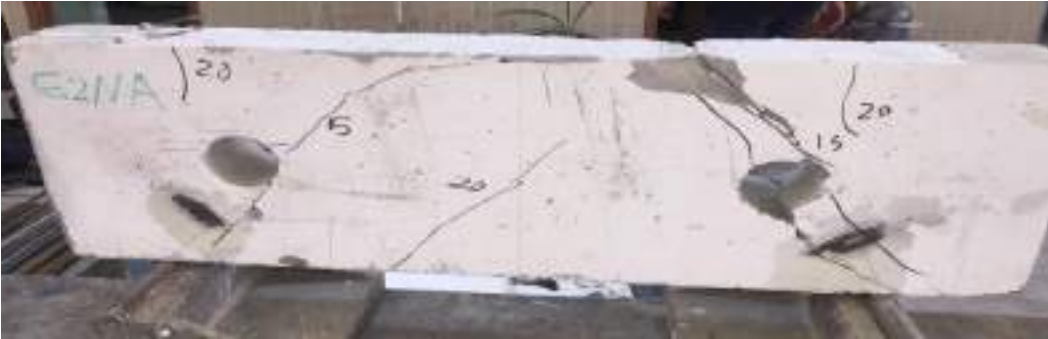
Plate (4.9) Experimental Deep beam G2NA1 (0%SF) after failure.
