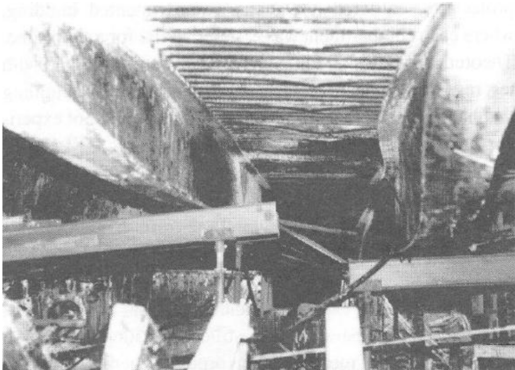
Figure (3-8): Considerable thermally induced beam [26].
