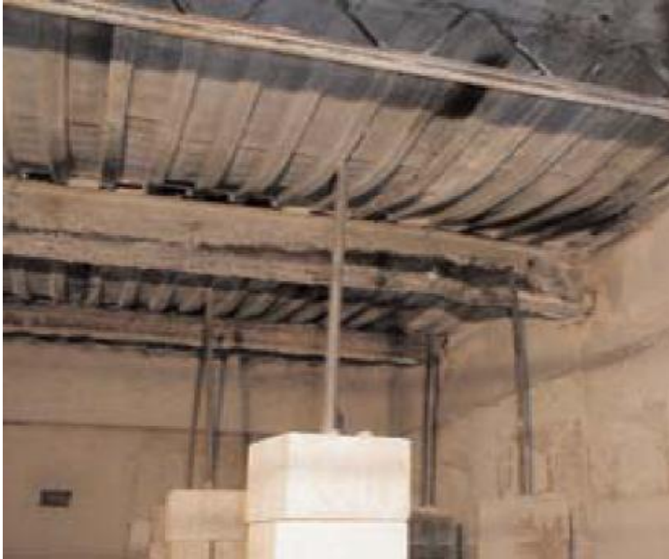
Figure (3-6): UL steel roof assembly after successful ASTM E119 fire test (courtesy of underwriters laboratories, Inc.) [29].
