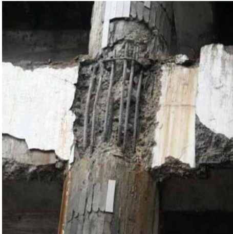
(a) Joint shear failure
