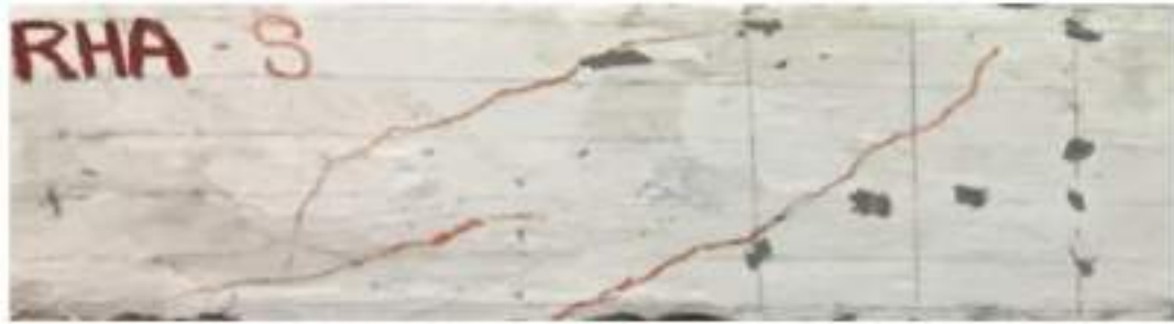
Fig. (2-4): Crack pattern for RH – marble powder of beam [40].
