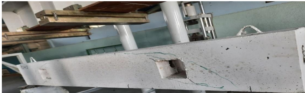
Figure 4.3 Load-deflection behavior and crack patterns for BW2.
