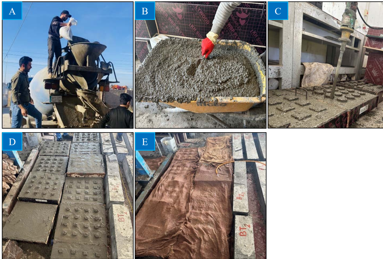
Figure 3.13 Casting and curing procedure of the specimens (A) loading raw materials into the concrete mixer, (B) concrete mix after mixing, (C) pouring the specimens, (D) specimens after pouring, (E), curing of specimens.
