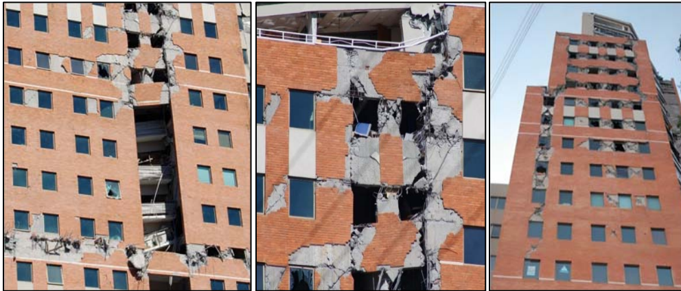
Figure 1.3 Shear failures of RC shear walls in Chile earthquake.
