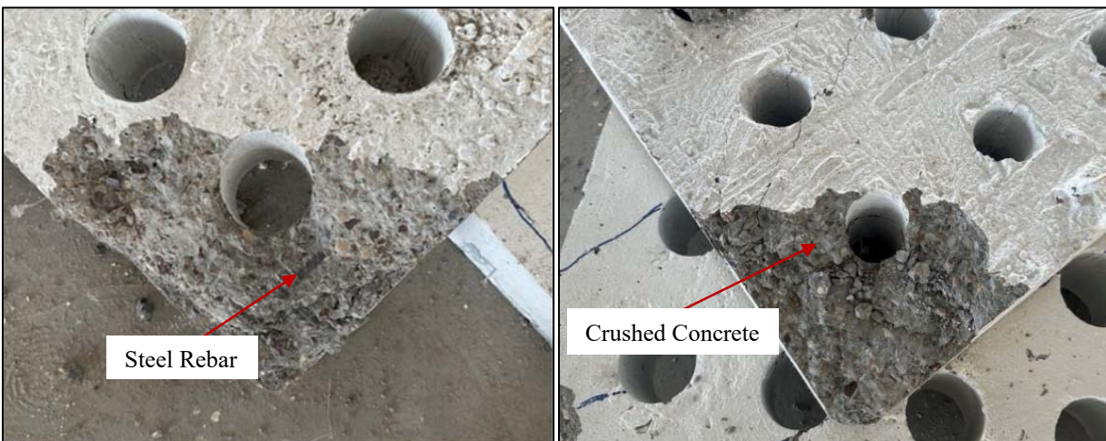
Figure 4.35 Crushed Concrete at loading area.
