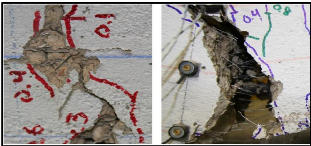
(a) Spalling at surface of concrete
