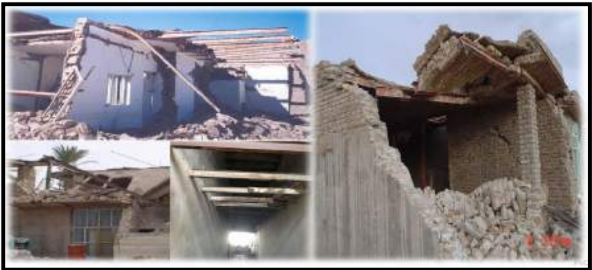
Figure. 1-4: Failure modes of masonry jack arch slabs [8].
