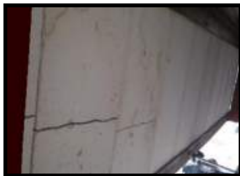
Figure 2-8: Failure in horizontal position [18].
