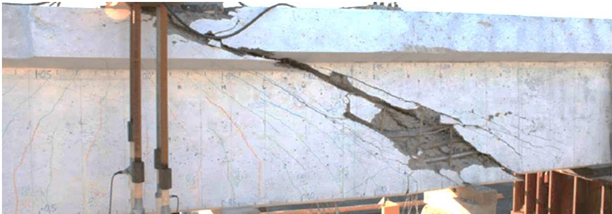
Figure 1.1 Diagonal shear crack [3].
