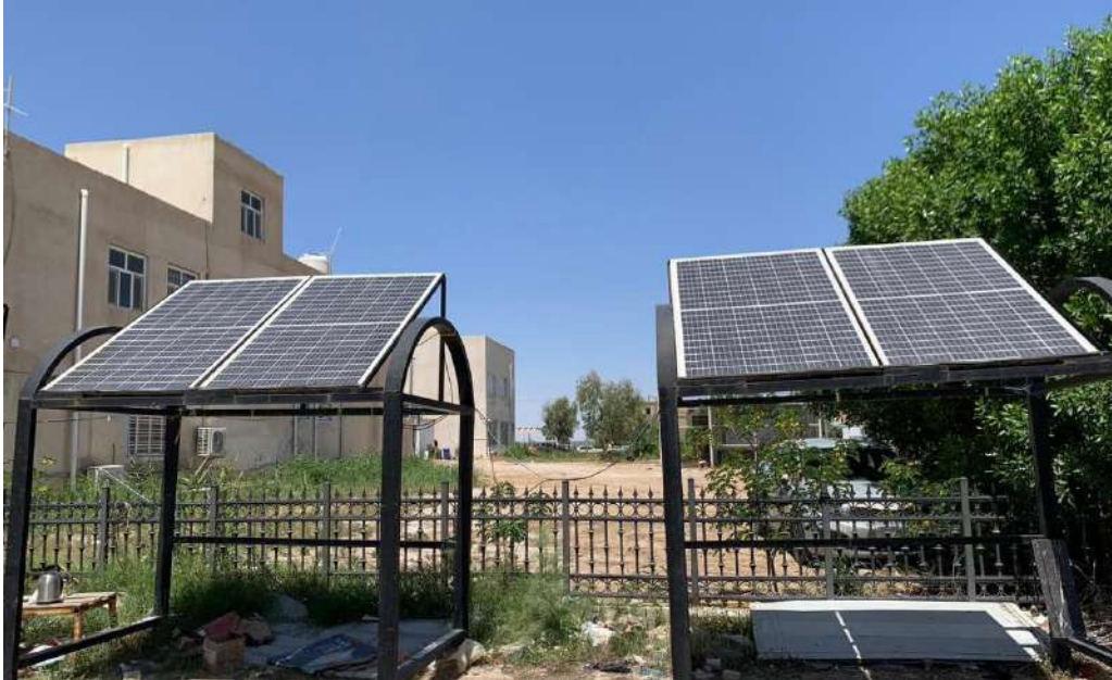
Figure 2-6 The outdoor PV system installed at the Engineering campus of University Misan, Iraq
