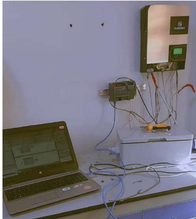
Figure 2-15 The computer connection to PLC to download PV power system data
