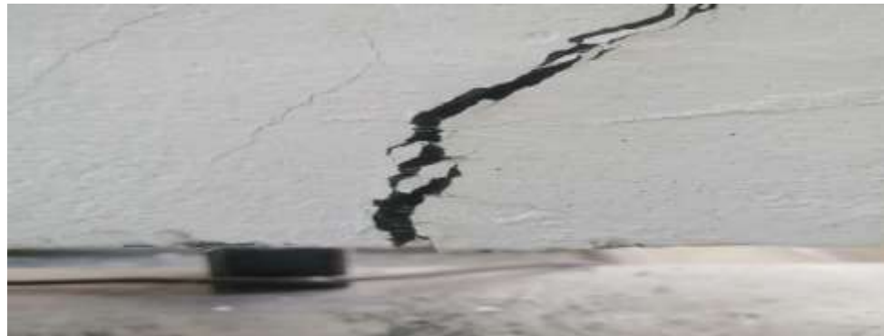
Figure 4.8 Crack pattern of MXB-4 (1% S.F).
