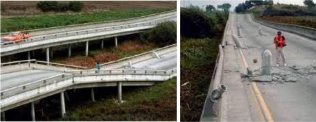
Figure 2. 2 bridge deck slab failing due to punching shear[29].
