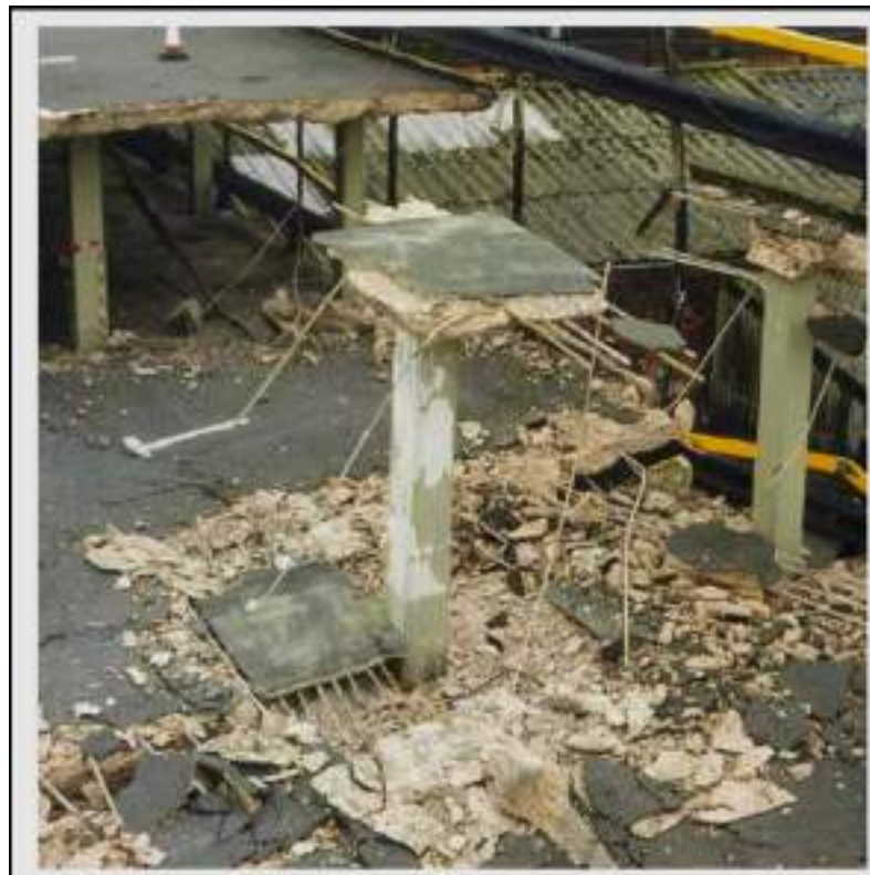
Figure (1.2) punching shear failure in Piper's Row Car Park, Wolverhampton, UK, 1997.
