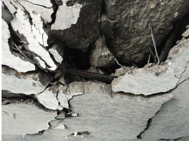
*Shapes of failure of slab specimen
