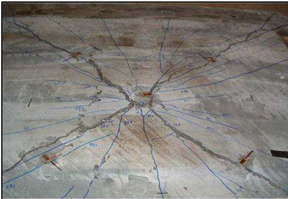
Plate (2-2): Typical slab failing in flexure[16].
