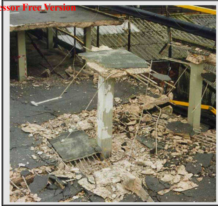
Plate(1-3): Punching Shear Failure in Piper's Row Car Park, Wolverhampton, UK, 1997 (built in 1965)[7].
