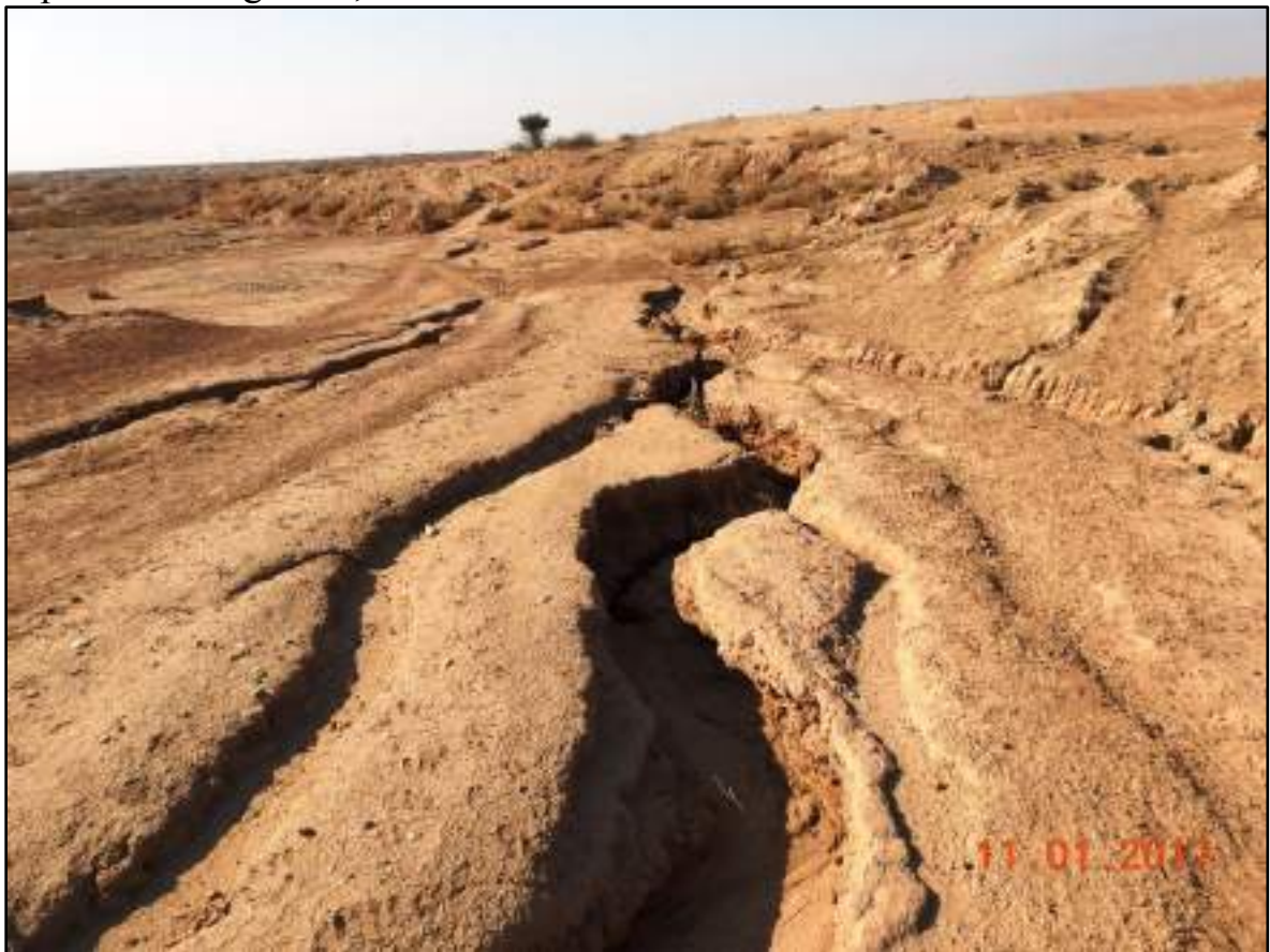
Fig. 5.17 Piping in soil of right shoulder
