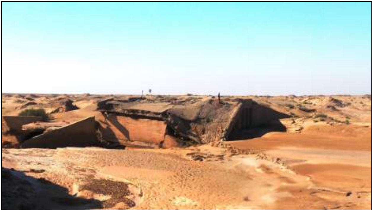
Fig. 5.14 Dispersive soil destroyed engineering structure (abridge) in study area
