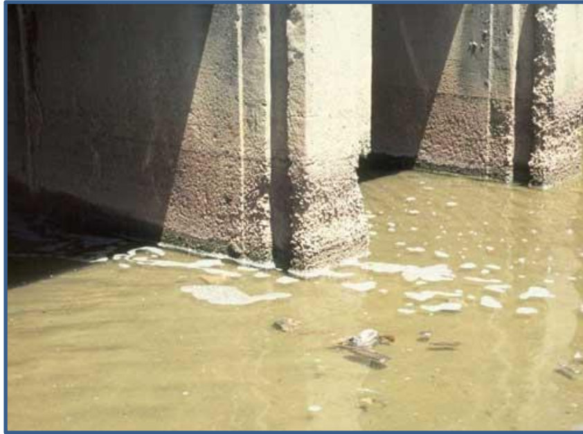
Fig.2.7 Effect of sulfates attack on hydraulic structure
