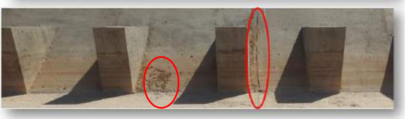
Fig.5.4 Effect of sulfates attack in dam slope, zone II
