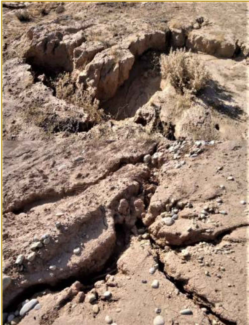
Fig.5.9 Grooves and gullies dispersive soil in left shoulder
