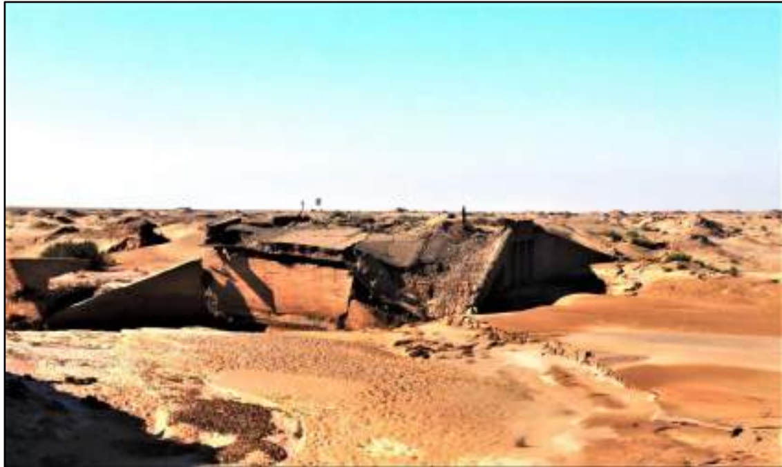
Fig. 5.10 Dispersive soil destroyed structure / abridge (Al-Sudani, 2018)
