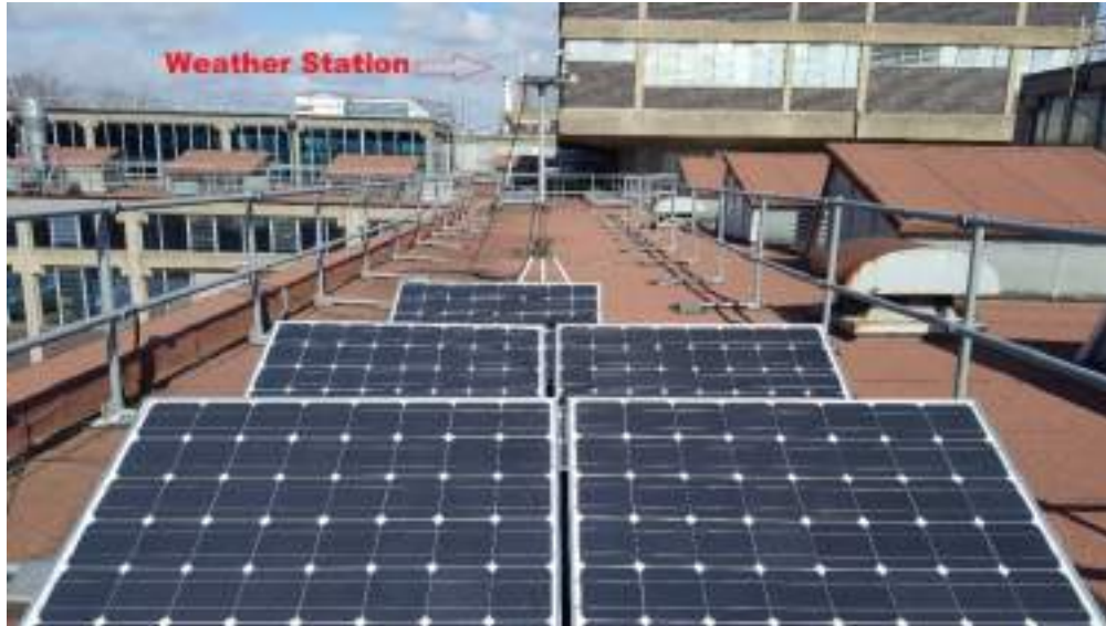
Figure 5.1. The studied PV array installed at Brunel University London, UK.
