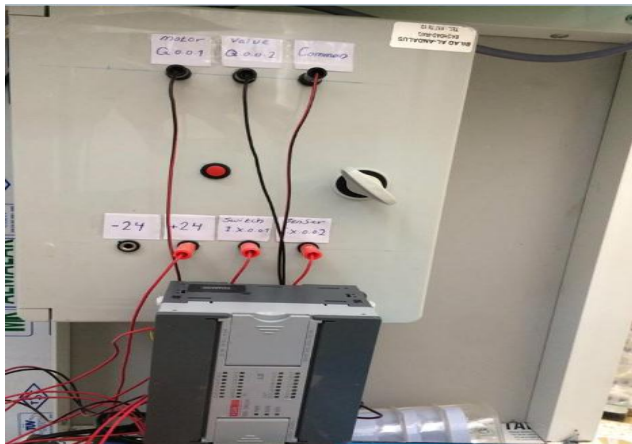
Fig-13: The Automatic control Panel.
