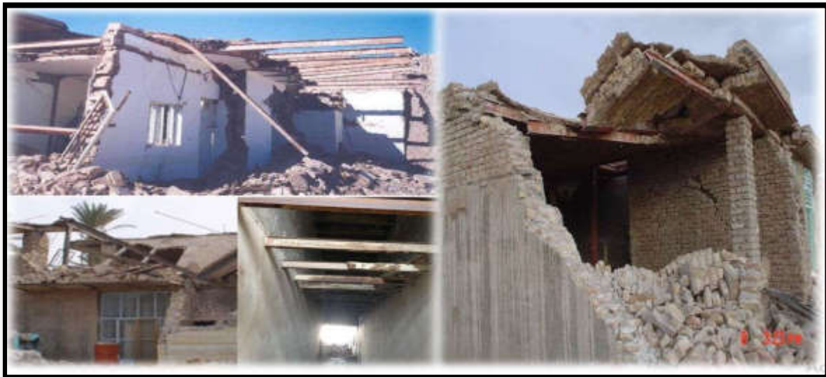
Figure. 1-4: Failure modes of masonry jack arch slabs [8].
