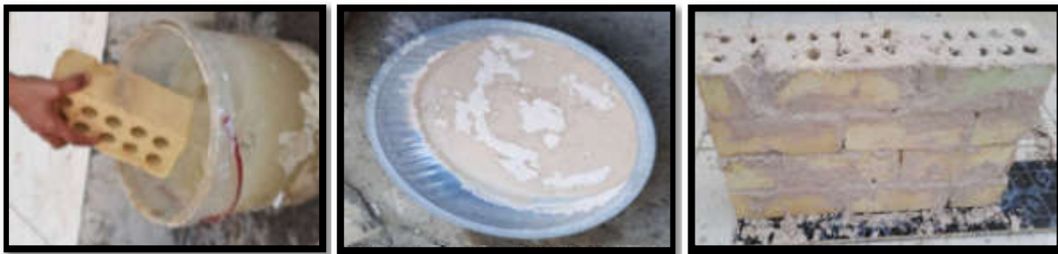
(a) Clean bricks.
