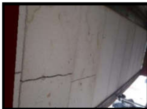
Figure 2-8: Failure in horizontal position [18].
