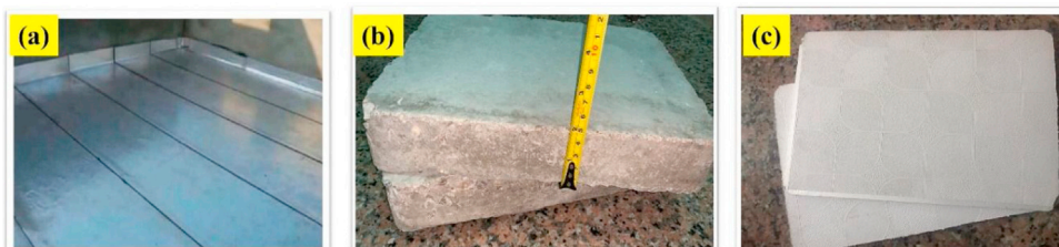
Fig. 2. Composite roof layers (a) photo for Isogam installation (b) concrete layers (c) gypsum boards.
